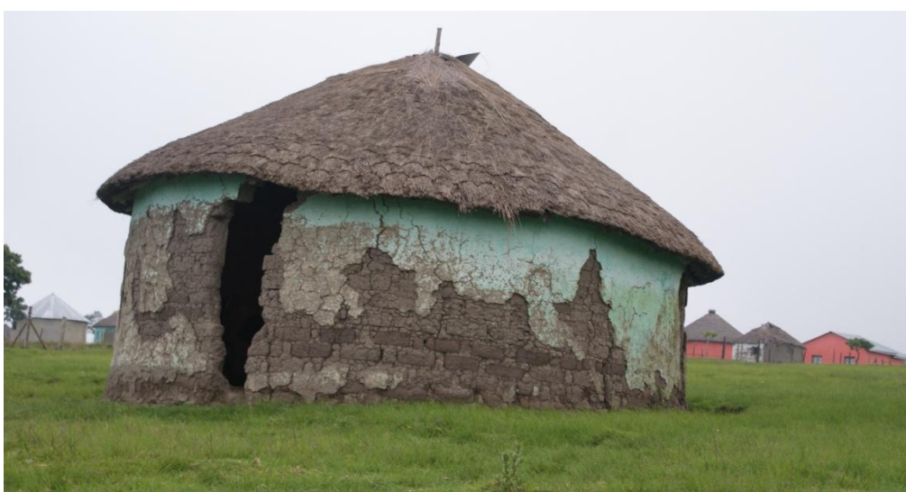
Dilapidated traditional rural dwelling
